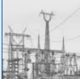
Air Insulated Switchgear
