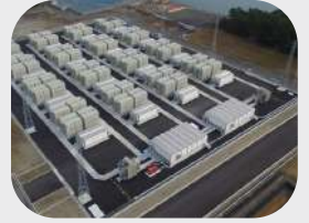
Battery storage stations
