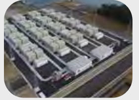
Battery storage stations
